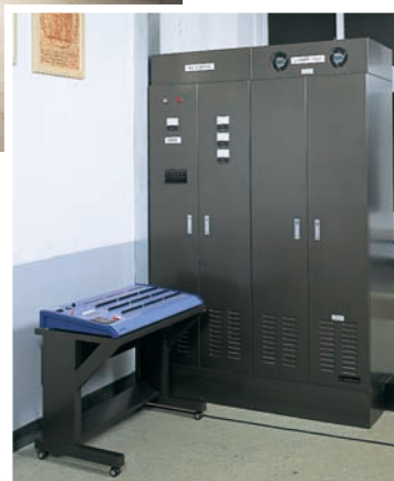
CONSOLE "LIGHTING BOARD" and DIMMER
